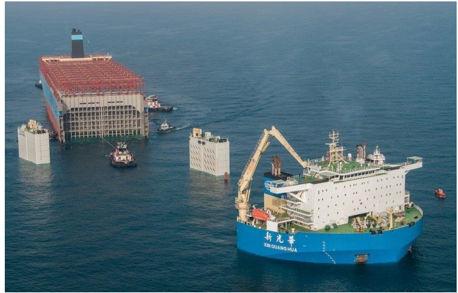
With bow and deckhouse removed, Maersk Honam's stern is loaded out for transport, 2018 (Maersk)
